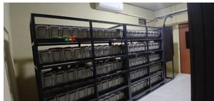
Battery bank — 2 × 50 × 12V 200Ah
