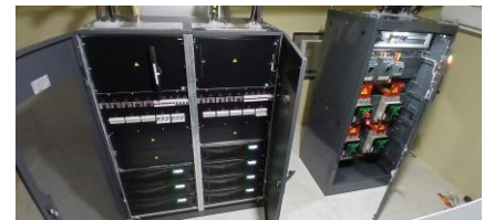
UPS modules — interior view
