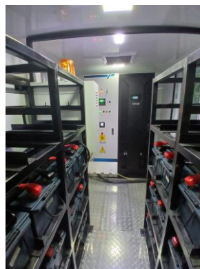
Interior — 100 KW (NTT)
